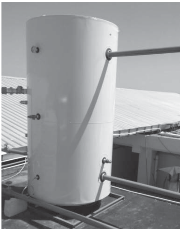
Solar-powered heater tank on SHMK rooftop
